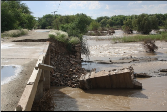
A severely damaged bridge on North Island
