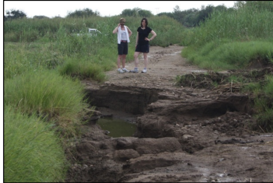
Water has swept away this road
