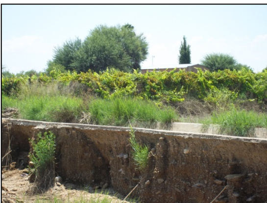
Irrigation channel at risk of collapse
